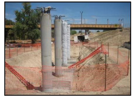
The new concrete bridge is supported on spread footings and four-column bents.
