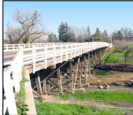
The original timber bridge, constructed in 1943, was demolished in 2008. Nineteen timber bents supported the 326-foot span. The new bridge will cross the creek with just five bents.
