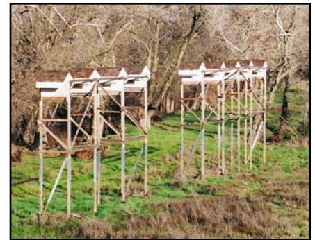
Nine prefabricated temporary roosting habitat for bats were lowered into place by helicopter.
