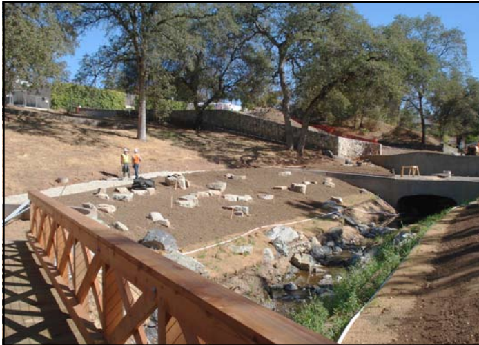
A new wooden pedestrian bridge is shown in the lower left foreground. Farther away, also on the left, two workers stand on the freshly-placed decomposed granite walking path. In the streambed, some of the freshly-planted vegetation is already sprouting. In the far background, more of the historic stone wall is visible.
