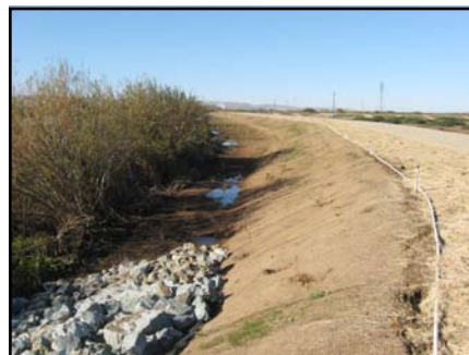
Erosion control mat installed on the newly constructed setback levee habitat bench.
