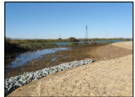
Setback levee habitat bench immediately after installation of erosion control mat and native plants.
