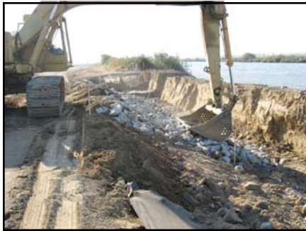
Installation of the riprap slope protection buried beneath the soil cover and native vegetation.
