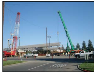
Erection was a dual crane process requiring both cranes to work in concert to place the girders weighing as much as 263,000 lbs.
